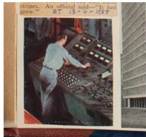
Image 2: Colour photograph of a man operating a control panel
